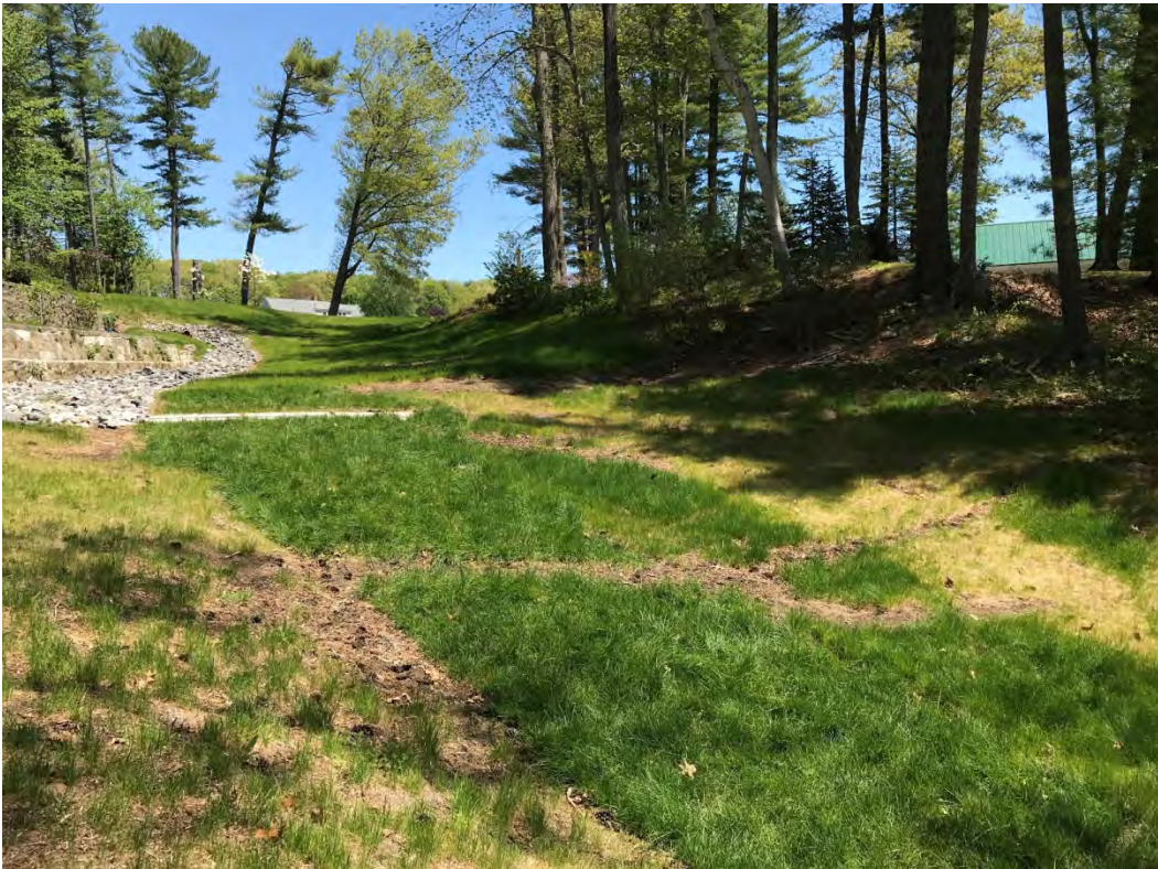
Fig 10: Slope below the manhole at Gundalow Landing/east side of the bay. Viewing east. (05-17-21)
