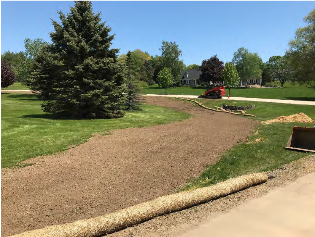
Fig 13: Loam spread over flowable fill work area at Gundalow Landing. Viewing east. (05-17-21)
