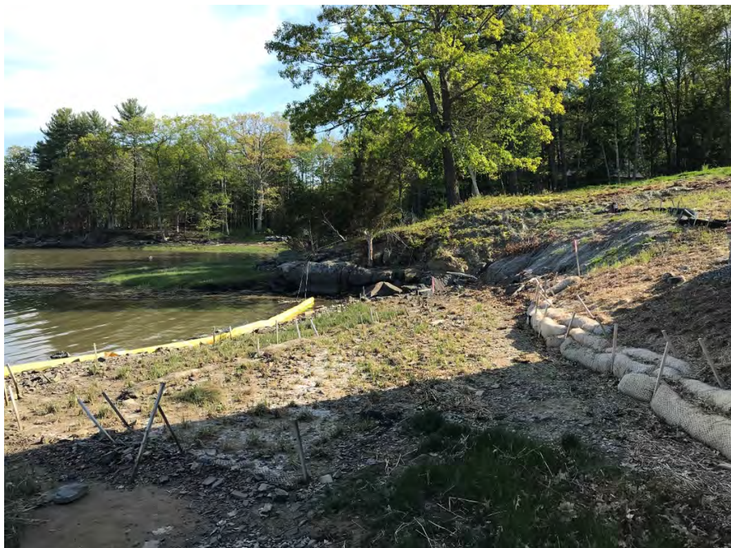
Fig 4: Toe of the slope and salt marsh restoration at the west side of the bay. Viewing south. (05-17-21)
